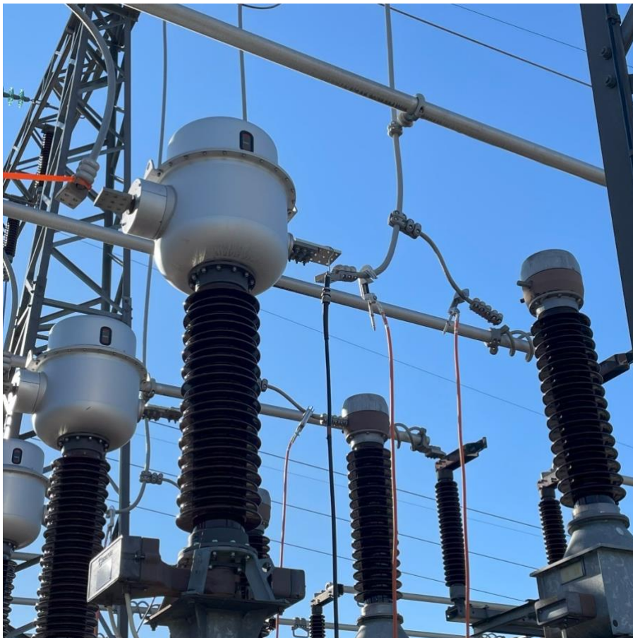
Figure 9. Measurement arrangements of the loss angle measurement. Current transformer being measured in the front left and voltage transformer on the right. Jumpers have been removed from primary terminals and orange grounding cords have been installed. Measurement voltage cable is hooked to the primary terminal of the CT.
