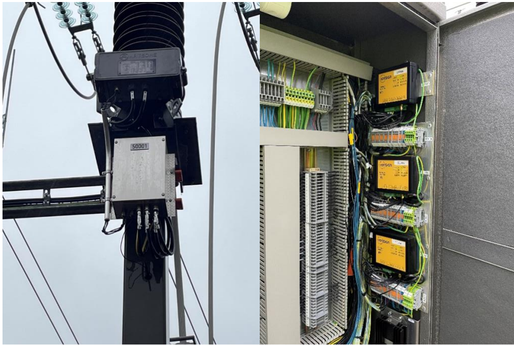
Figure 12. IoT5 device installed on the CT leg (left) and IoT5 devices installed inside the distribution cabinet for every three phases (right).
