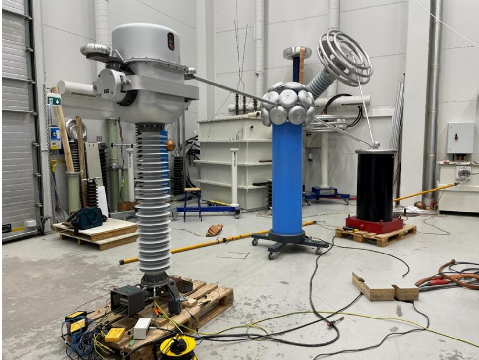
Figure 16. Measurement arrangement for the new CT. In the foreground, the current transformer to be measured, the yellow IoT devices connected to it, and the white measuring bridge signal connection box. The current transformer is connected with a busbar to a blue compressed gas capacitor, which in turn is connected to a black voltage transformer. The voltage transformer is connected to the test transformer, which creates the voltage. The reference voltage for the IoT devices is brought from the voltage transformer with the black cable.
