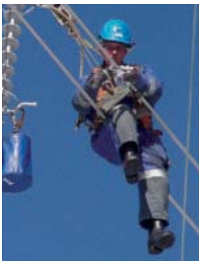
Conductors being installed on the Varkaus - Huutokoski line site in December 2003. Veli Ikonen at work.
