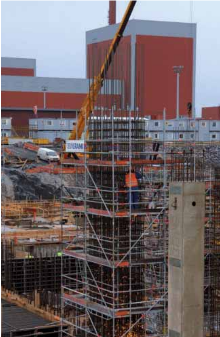
The third unit at the Olkiluoto nuclear power plant is due to be ready by the turn of 2010 and 2011. For Fingrid, the technical solutions, arrangements and capital investments for connecting the unit to the grid have progressed as planned; the new transmission lines and substations will be complete by the end of 2008.
