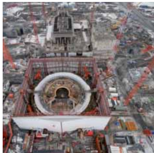
The construction site of the third nuclear power plant unit at Olkiluoto is moving over to the installation of main machinery. Work is carried out in three continuous shifts.
