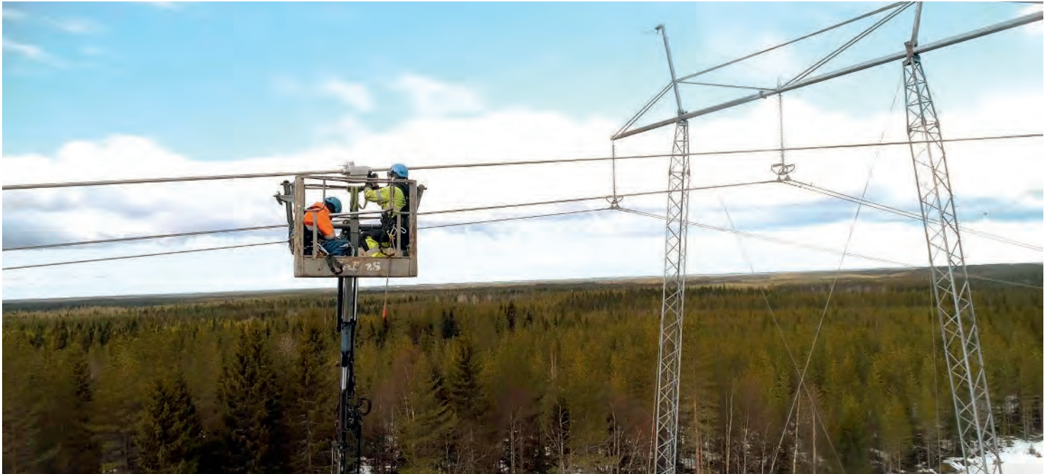
The installation of sensors for DLR systems on the Isokangas–Pyhänselkä line near Oulu was carried out last spring. Four different sensors were installed on sections that are considered critical in terms of thermal loading.
