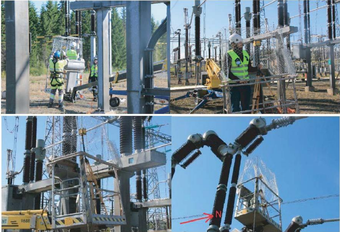
Figure 3-21 Photos of the Faraday cage installed on a man hoist.
