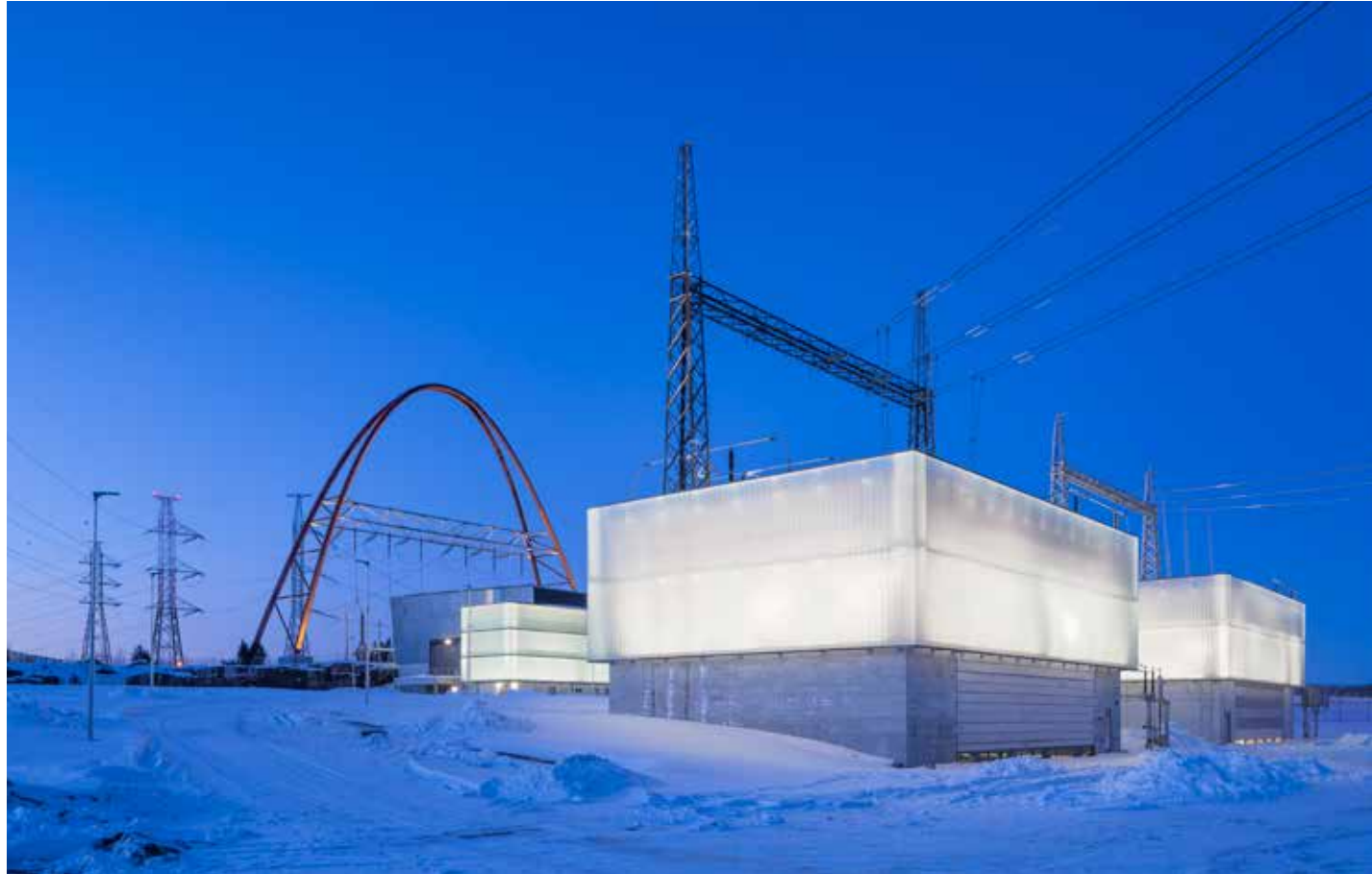
The substation in Länssalmi, Vantaa, has been expanded from a single transformer bay to a four-bay switchgear plant.
